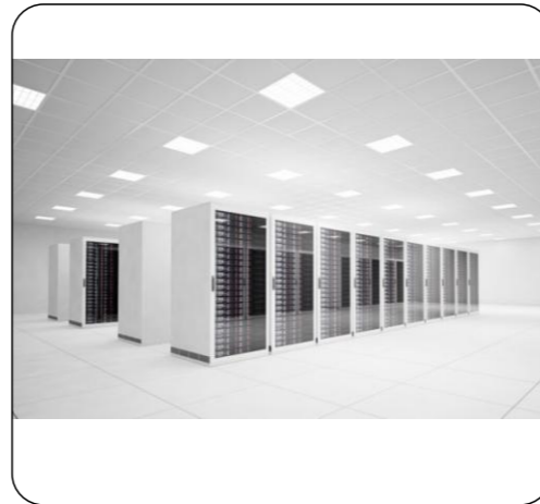
[ Multiple Diverse Data Processing Sites ] [ System is fully distributed and is not dependent upon any single site or component Seamless and secure remote access to all hardware, software and services Multiple data centre providers to further enhance diversity ]
